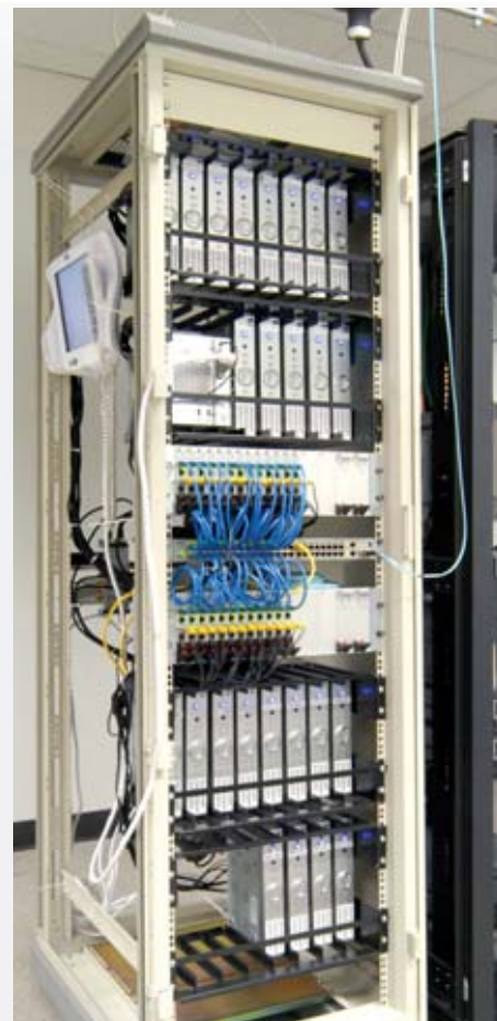
IPTV head end with rack-mounted satellite receivers (the silver boxes) and Visionary Solutions encoder blades (behind and below the blue patch cables).
