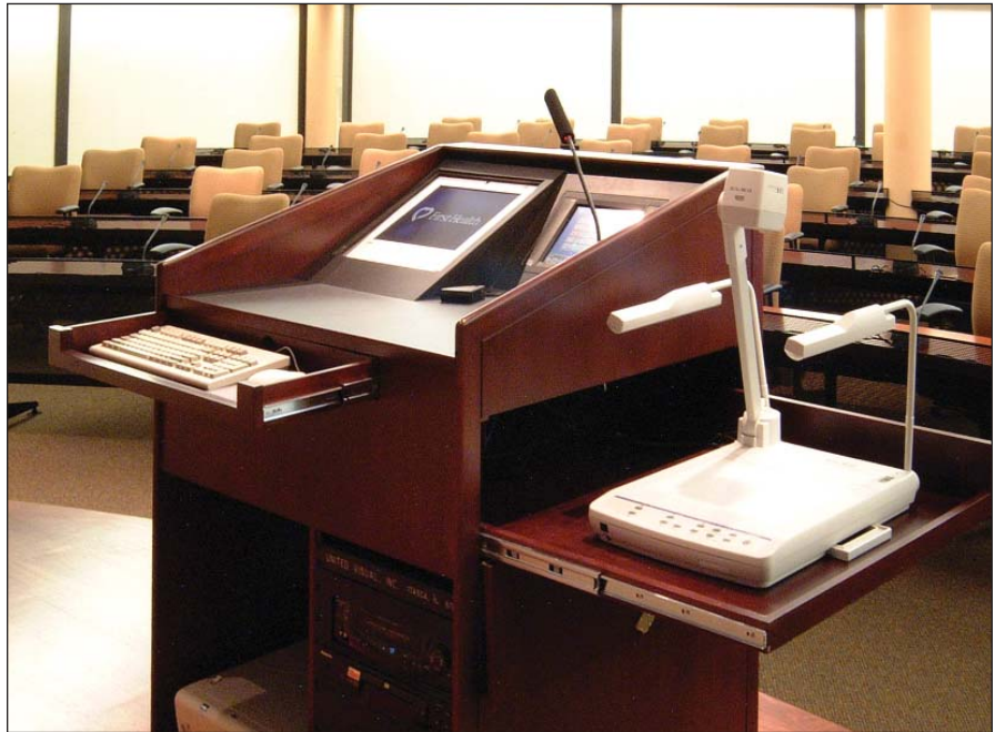
Above: presenters in First Health's auditorium can control all systems themselves from this podium, or they can rely on technicians working out of an operators' area on the side of the room (shown on the cover).
