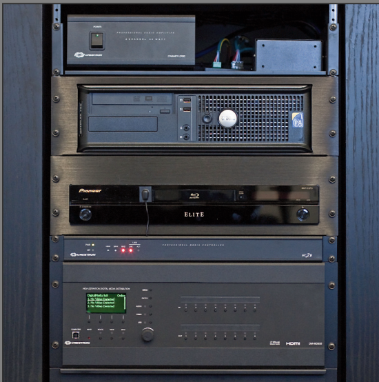
Equipment rack in the Presentation Room, with Crestron DM-MD8X8 DigitalMedia switcher, MC2E processor, CNAMPX-2X60 amplifier, plus Pioneer Elite Blu-ray player and Dell Optiplex computer installed.
